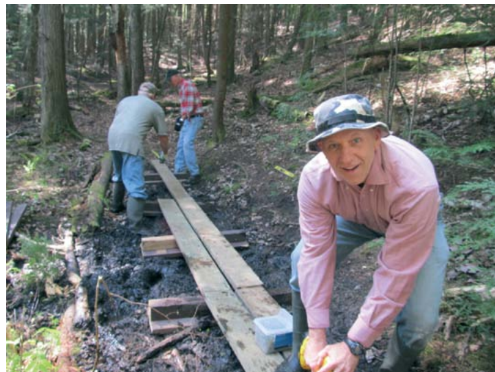
Tim drills deck screws while David and Larry lay out the next section.
